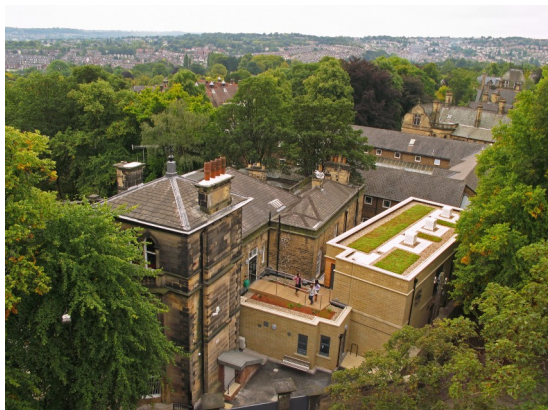
Our New Sixth Form Extension is now complete and the girls were welcomed on the first day of term to the new facilities with banners, balloons and bacon butties!
